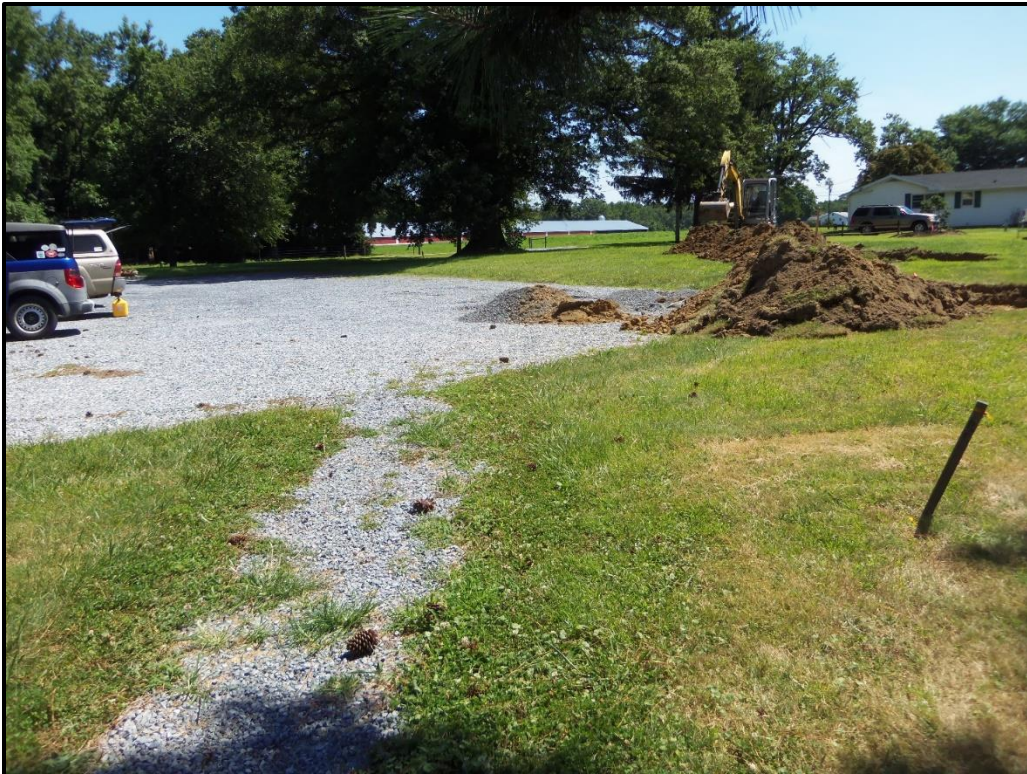
Figure 9. Trench excavation from the southwest corner of the parking lot toward the northeast
